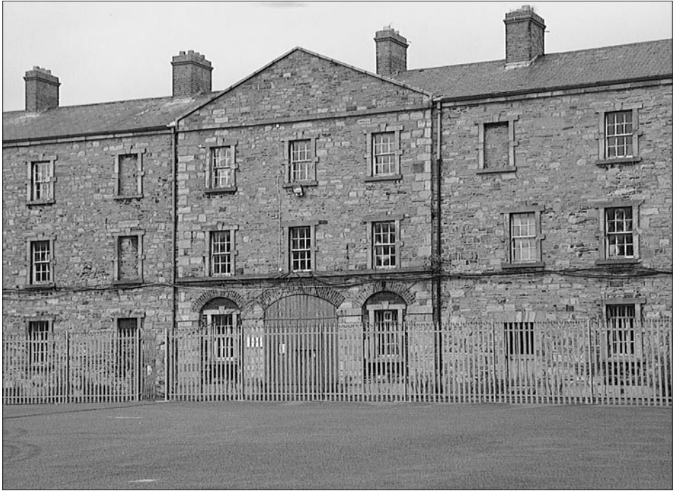
4 – Thomas Burgh, centre block of Horse Square (begun 1703), Royal (Collins) Barracks, Dublin The original walling material – calp limestone rubble with limestone quoins – is clearly visible, as are the granite window dressings introduced in Thomas Eyre’s reconstruction of 1758-59.
