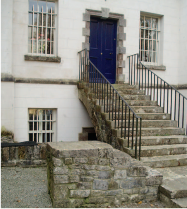
4 – A mounting block in the stable yard at Ardraccan, Co Meath (photo: the author)
