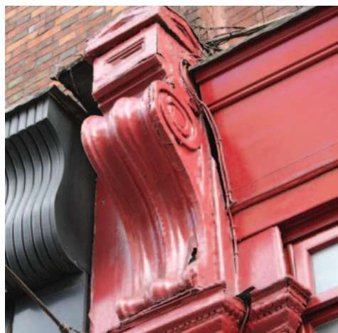
15 – Bracket detail to the shopfront of the first range of buildings between Grand Parade and South Main Street at 3 Washington Street
