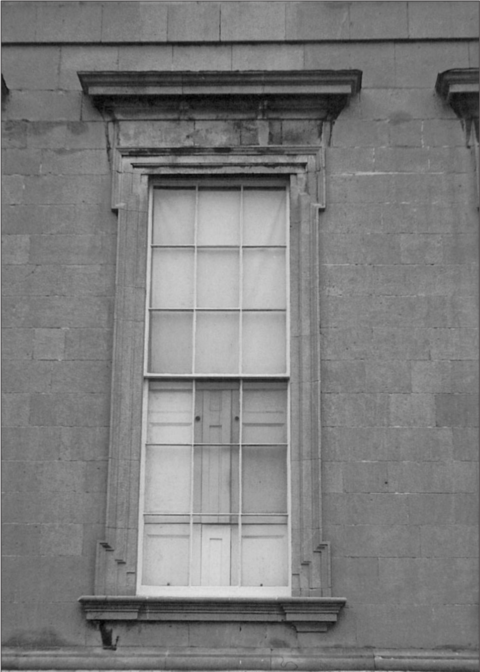
1 – Castletown, Co Kildare – clerestory window in hall showing the impressionistic effect of crown glass (photo: the author)
