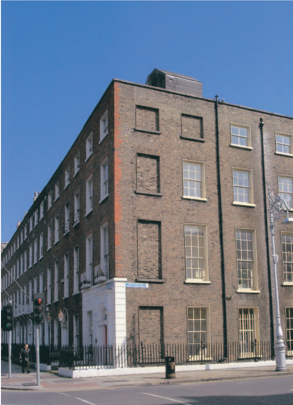
1 – Blind windows on Upper Mount Street, Dublin (all photos by the author)
