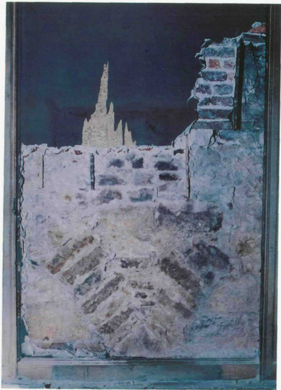
5. Main Guard, Clonmel. Segments of two relieving arches interrupted by insertion of present first floor windows.
