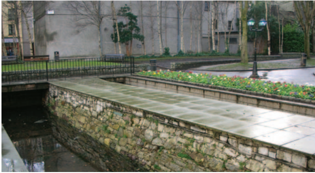
7 – Excavated lower section of city walls at Bishop Lucey Park, Grand Parade, Cork (incorporating seventeenth-century repairs)
