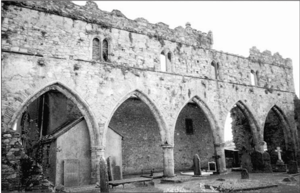
14 – St Mary's, Thomastown: view from the north showing the north aisle arcade with the new church and vestry in the nave
